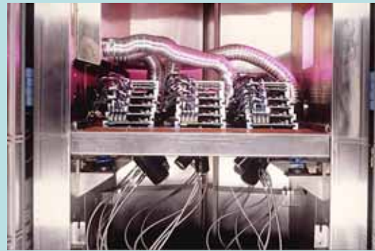
Figure 25-45 Flexible Air Ducting
